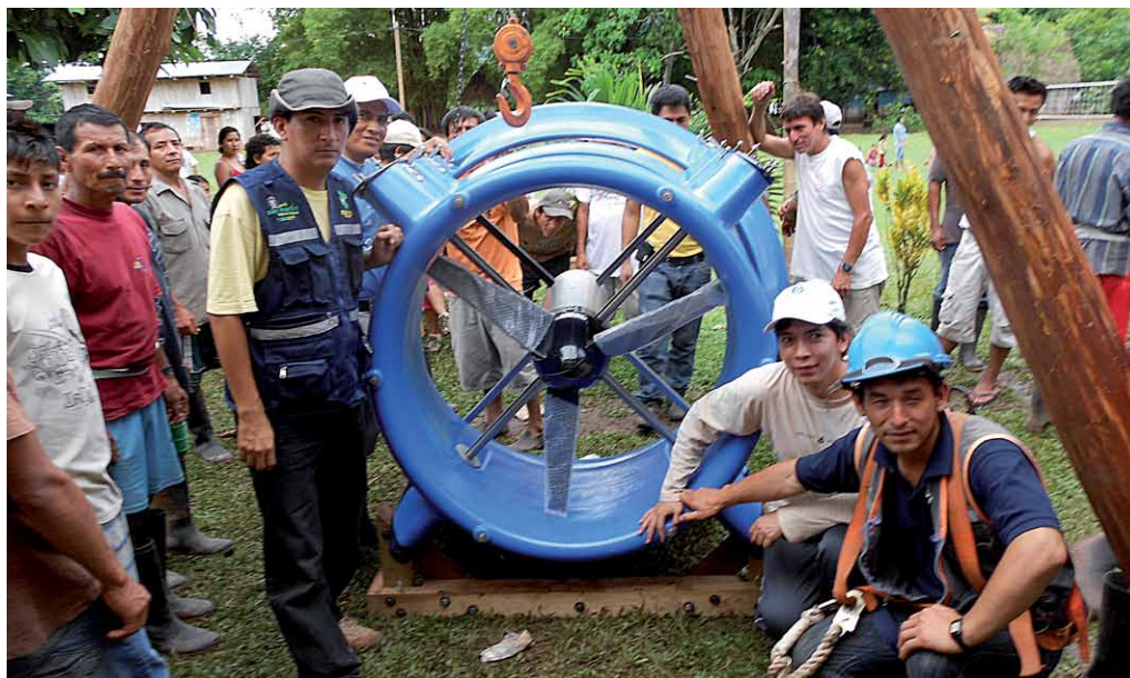
The turbine just before its installation in Marisol. © Smart Hydro Power
