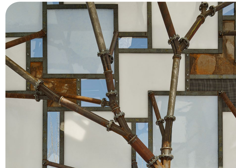
The steel frame of the pavilion looks like a tree. Courtesy of Zoey Brown.
