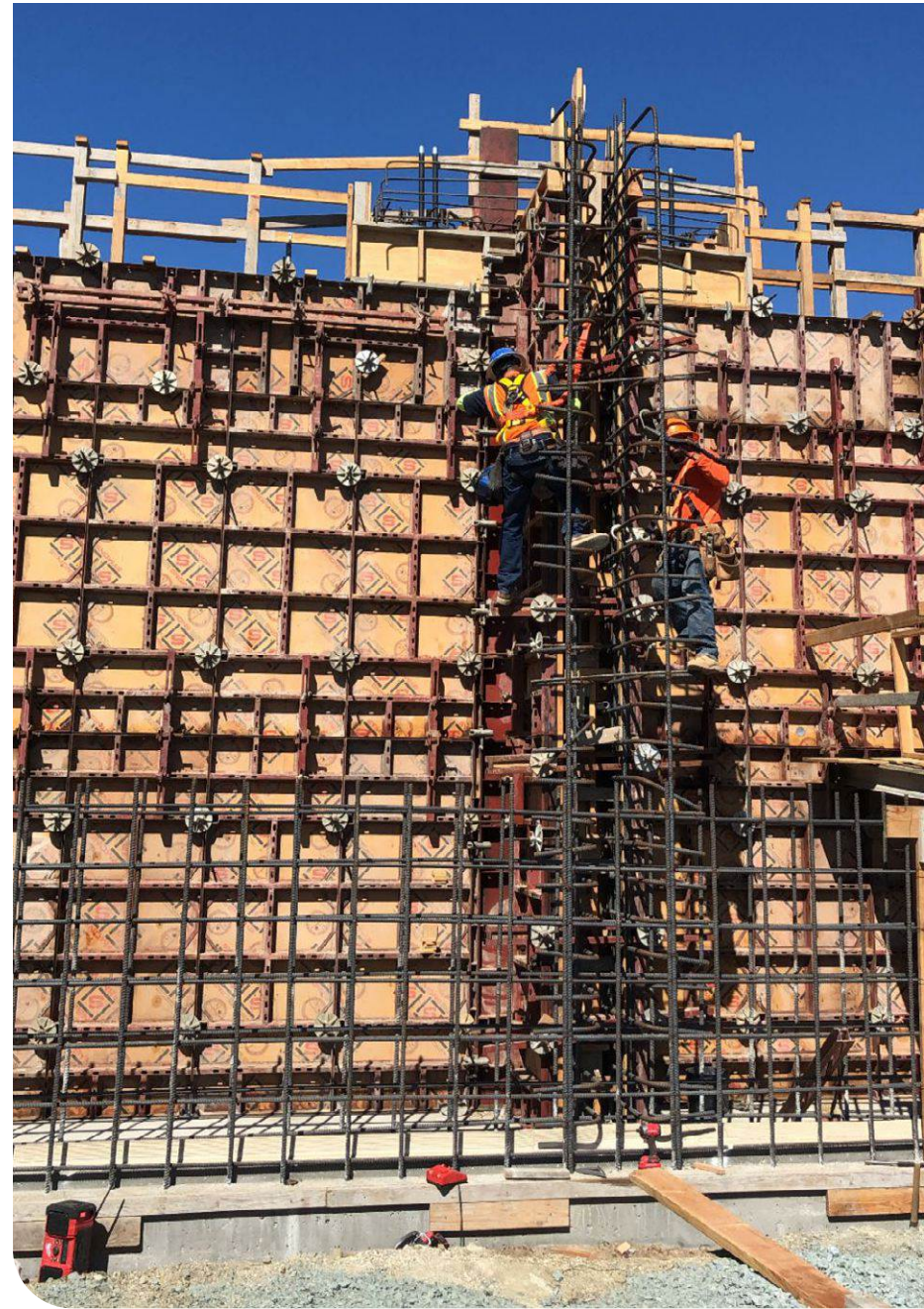
The new facility will help Morro Bay discontinue the discharge of treated wastewater to the ocean and create a new sustainable and local water resource. Courtesy of City of Morro Bay.
