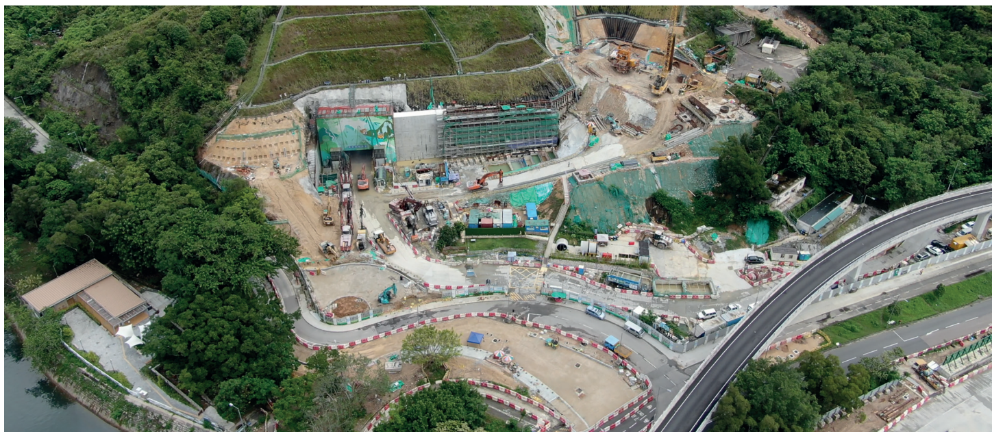
Site Photo of Relocation of Sha Tin Sewage Treatment Works to Caverns (Stage 1 Works)
