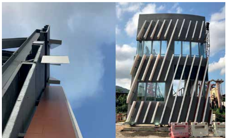
Visual Mock-up for Design Review & Kinetic Effect Simulation Image Courtesy of Hip Hing Engineering Company Limited and Architectural Services Department, HKSAR Government and Vircon Limited
