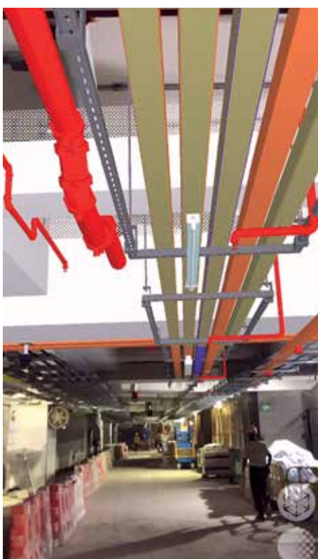
AR technology had helped the BIM adoption on the construction site. Image Courtesy of Gammon Construction Limited and Hong Kong Science and Technology Parks Corporation
