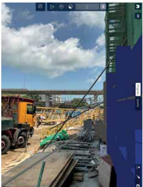
Augmented Reality (AR) with BIM Image Courtesy of Airport Authority Hong Kong and China State Construction Engineering (Hong Kong) Limited
