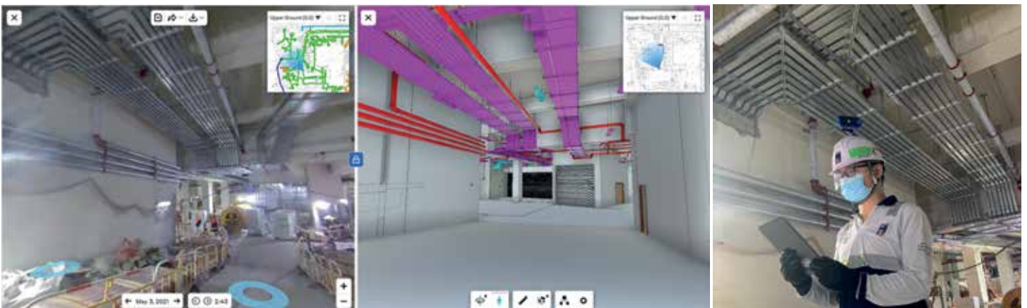
Daily project reality capture via 360 camera allowing for model comparison to existing work Image Courtesy of Leighton Contractors (Asia) Limited
