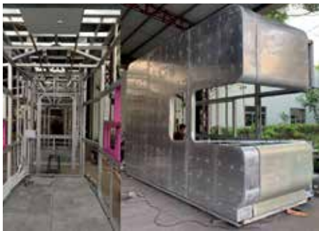
Off-site_MiC Prefabrication Image Courtesy of Hip Hing Engineering Company Limited and Architectural Services Department, HKSAR Government and Vircon Limited
