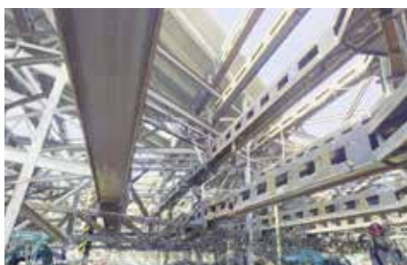
3D laser scanning technology enhanced the speed and accuracy of data collection from construction sites Image Courtesy of Airport Authority Hong Kong and China State Construction Engineering (Hong Kong) Limited
