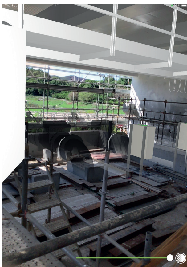
AR Application on Site Image Courtesy of Drainage Services Department, HKSAR Government and AECOM Asia Company Limited and The Jardine Engineering Corporation, Limited
