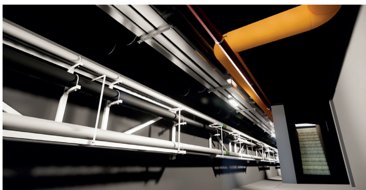
Design for Manufacture and Assembly (DfMA) of Tunnel Services Gallery Image Courtesy of Gammon Construction Limited
