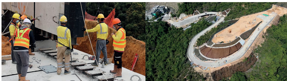
Lifting and assembly of retaining wall; Overview of retaining wall Image Courtesy of Drainage Services Department, HKSAR Government and AECOM Asia Company Limited
