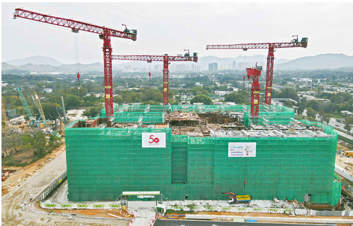
Overall Bird View, Pioneer MiC project located in Kwu Tung North Image Courtesy of Architectural Services Department, HKSAR and Shui On Joint Venture and Vircon Limited
