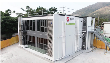
First Run of MiC Mock up and lifting for future MiC Installation Image Courtesy of Architectural Services Department, HKSAR and Shui On Joint Venture and Vircon Limited
