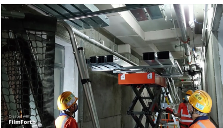
Cycle Installation of trunking by Multi-trade Integrated MEP (MiMEP) in MiC corridor Image Courtesy of Architectural Services Department, HKSAR and Shui On Joint Venture and Vircon Limited
