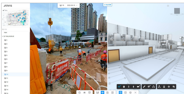
Construction Monitoring (Eagle Eye System) Image Courtesy of CLP Power Hong Kong Limited
