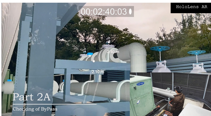
Augmented Reality (AR) - Design Verification Image Courtesy of Electrical and Mechanical Services Department, HKSAR
