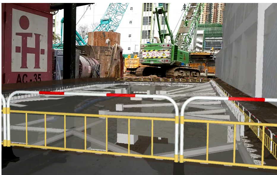
Visualize the ELS works model at site by AR. Image Courtesy of Architectural Services Department, HKSAR and Shui On Joint Venture
