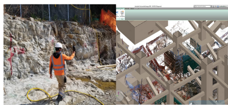
Surveying with 3D handheld scanner seamlessly integrating site condition into the BIM model. Image Courtesy of Architectural Services Department, HKSAR and Shui On Joint Venture and WSP Hong Kong Limited
