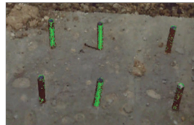
Scan imagery of misaligned rods
