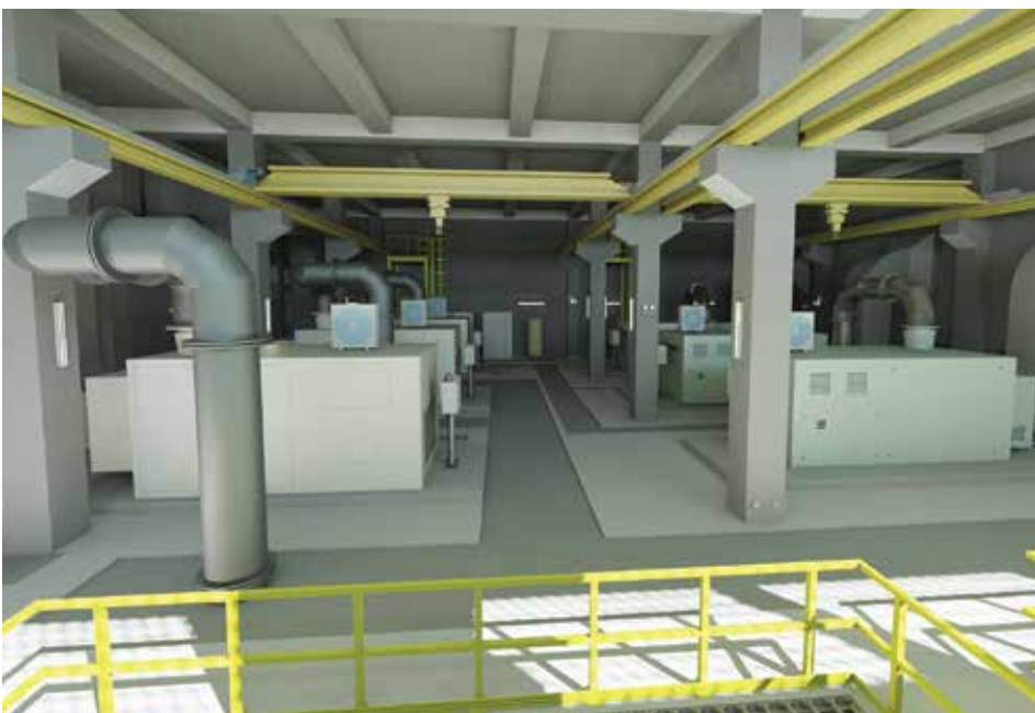
Internal view of the Membrane Facilities Building with Air Scouring Blower and Aeration Blower for backwash Image courtesy of Drainage Services Department, HKSAR Government and Summit Technology (Hong Kong) Limited
