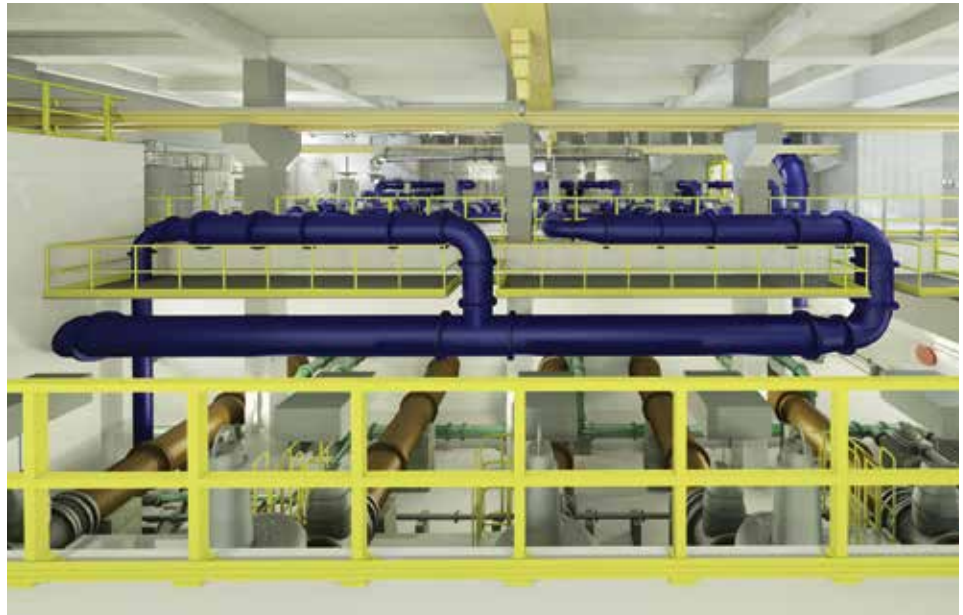
Internal view of the Membrane Facilities Building where the treated water exits from the membrane filters Image courtesy of Drainage Services Department, HKSAR Government and Summit Technology (Hong Kong) Limited
