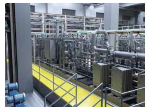
On-site Chlorine Generation Skids with Walkways for Operation and Maintenance Access Fitted within Chlorine Store using BIM Model to Optimize Space Utilization Image courtesy of Water Supplies Department, HKSAR Government
