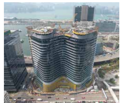
Bird's eye view of The Quayside from Wai Yip Street Image courtesy of Link Real Estate Investment Trust and Nan Fung Development Limited
