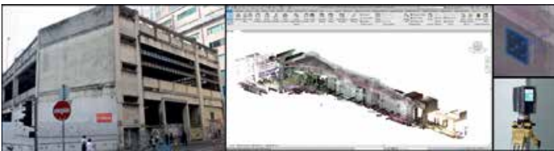
Demolished KMB Depot and Laser Scanning for Curtain Wall Fabrication Image Courtesy of Yee Fai Construction Company Limited
