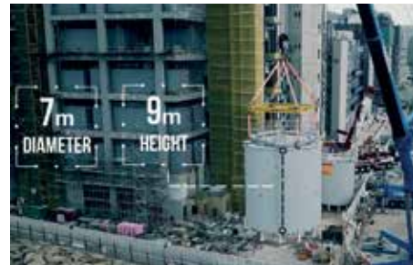
The MiC thermal tank weighted 50 ton each being just-in-time installed to the site. Image Courtesy of Global Switch
