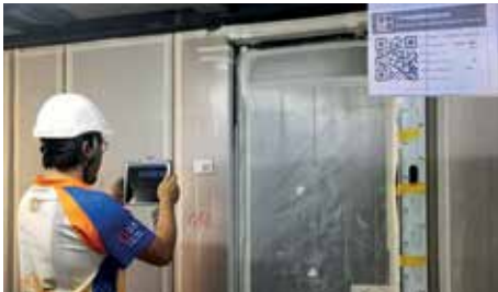
QR code scanning and QA/QC inspection Image Courtesy of Hip Hing Engineering Company Limited and Architectural Services Department, HKSAR Government
