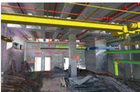
Point Cloud 3D Scanning Imposing BIM for Site Verification and Measurements Image Courtesy of Drainage Services Department, HKSAR Government and AECOM Asia Company Limited and ATAL-Degremont-China Harbour Joint Venture
