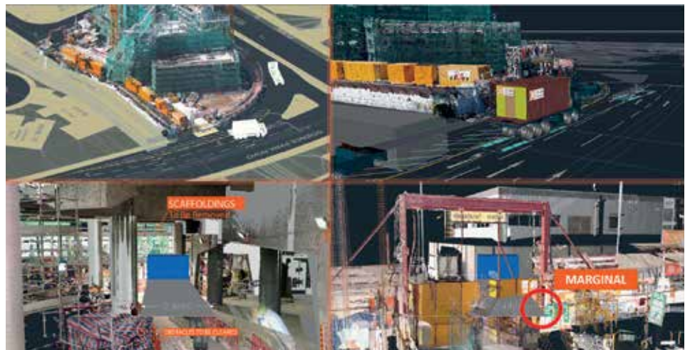
Swept Path Simulation of Module-Loading Vehicle Along the Site Image Courtesy of Hip Hing Engineering Company Limited and Hong Kong Science and Technology Parks Corporation and Leigh & Orange Limited
