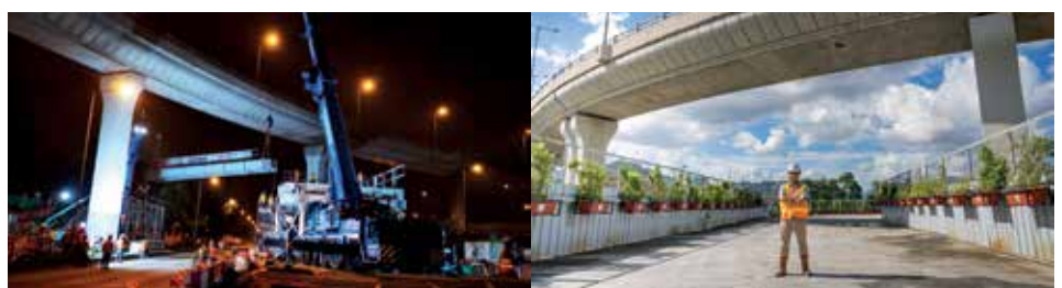
Lifting of the bridge deck segments at night and completed steel bridge Image Courtesy of Drainage Services Department, HKSAR Government and AECOM Asia Company Limited
