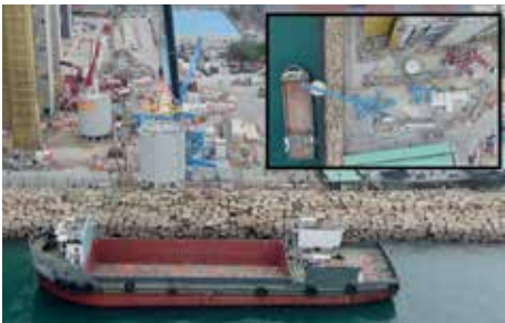
Hoisting operation of the heaviest MiC thermal tank in Hong Kong. Image Courtesy of Global Switch
