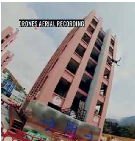
Daily construction progress record by drone Image Courtesy of Hip Hing Engineering Company Limited and Architectural Services Department, HKSAR Government
