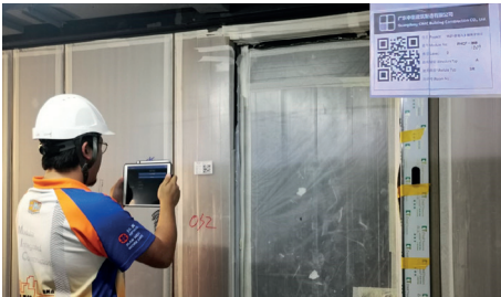
QR code scanning and QA/QC inspection Image Courtesy of Hip Hing Engineering Company Limited and Architectural Services Department, HKSAR Government
