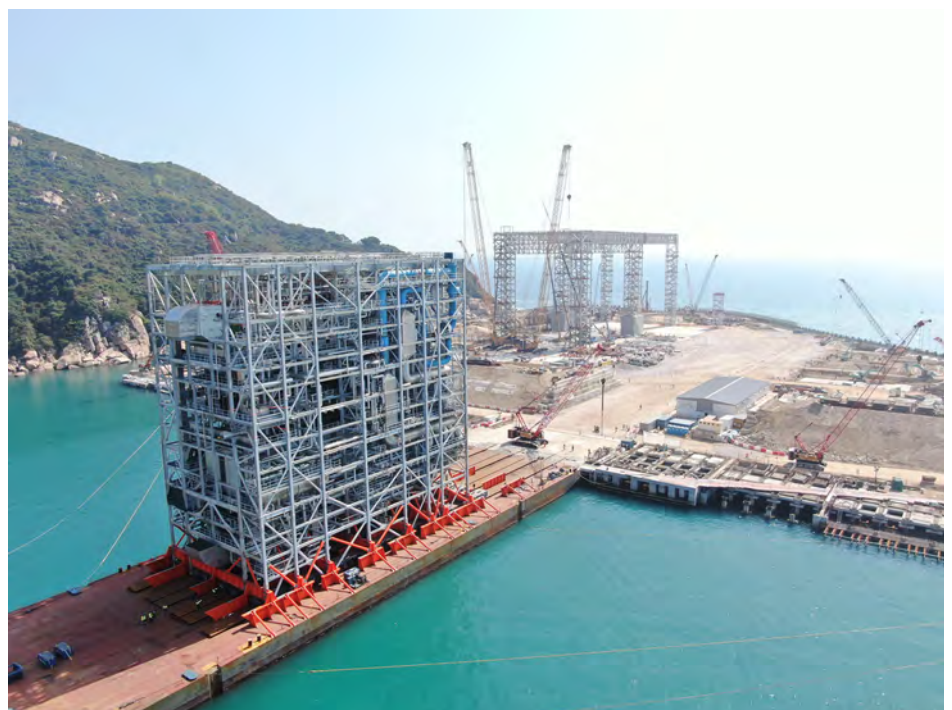
Actual MiC unit Delivery on site Image Courtesy of Environmental Protection Department, HKSAR and China Harbour Engineering Company Limited and Keppel Seghers – Zhen Hua Joint Venture
