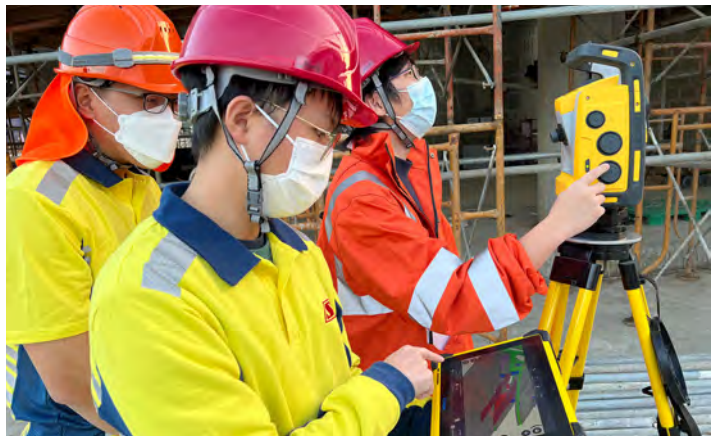
Technology adoption - Robotic Total Station Image Courtesy of Sun Hung Kai Properties Limited and Sanfield (Management) Limited and Strategic Building Innovation (SBI) bimSCORE Limited
