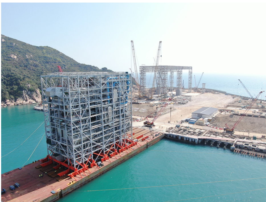
Actual MiC unit Delivery on site Image Courtesy of Environmental Protection Department, HKSAR and China Harbour Engineering Company Limited and Keppel Seghers – Zhen Hua Joint Venture
