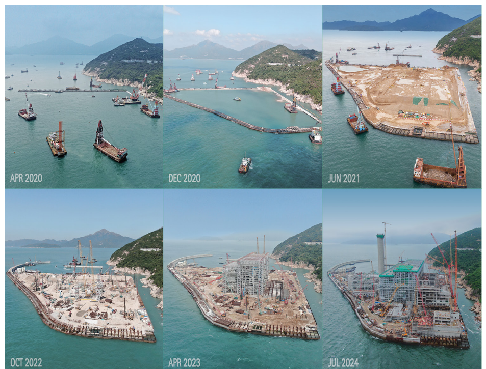
Project Progress Photo Image Courtesy of Environmental Protection Department, HKSAR and China Harbour Engineering Company Limited and Keppel Seghers – Zhen Hua Joint Venture
