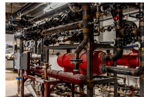
Fluid systems and fluid power equipment
