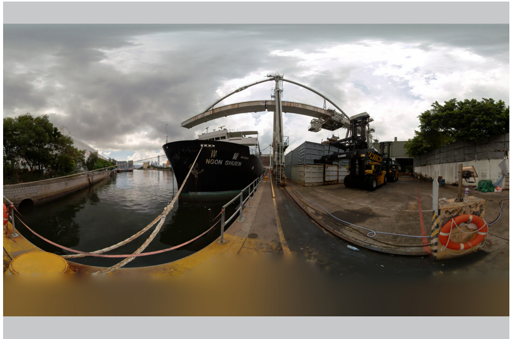
Panoramic image capturing for gantry crane dismantling and installation Image Courtesy of Environmental Protection Department, the Government of the Hong Kong Special Administrative Region & AECOM Asia Company Limited & China Harbour Engineering Company Limited
