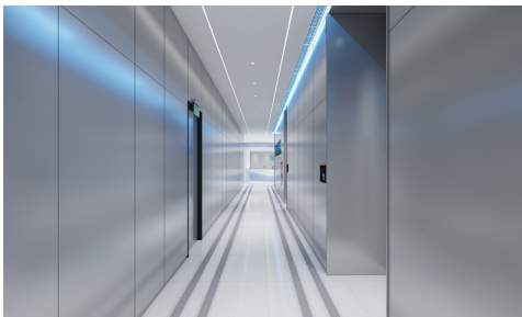
Data Services Platform (DSP) Image Courtesy of Hong Kong Cyberport Management Company Limited
