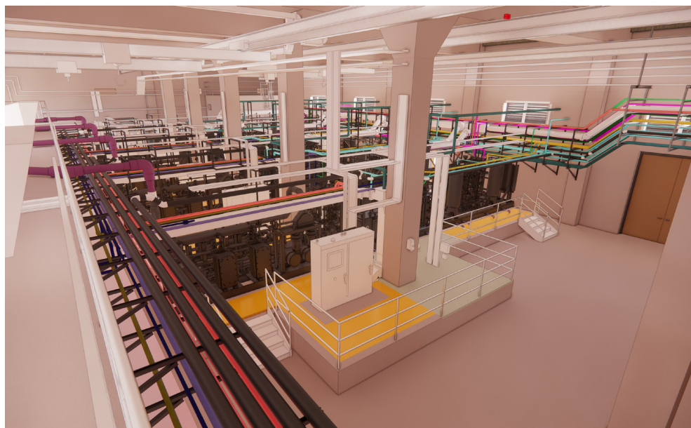
Overall View of Tai Po WTW OSGC BIM As-built Model Image Courtesy of Water Supplies Department, the Government of the Hong Kong Special Administrative Region and Shenzhen Yuegang Technology Co., Limited and The University of Hong Kong, HKU Business School
