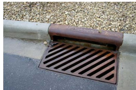
Storm sewer catch basin intake structure (Neenah casting). Image courtesy of Bolton & Menk, Inc.
